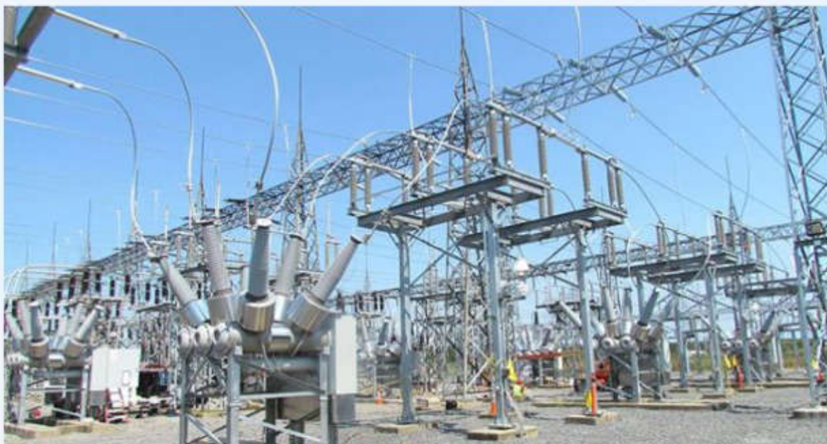
Figure 2: The electrical grid in Ghana has adequate capabilities to integrate NEK's wind energy projects into the power mix and the 330 kV WAPP transmission line also allows for exports into neighbouring countries. (Picture source: https://www.cedidollar.com/ghana-receives-e9-7m-eu-grant-to-improve-access-to-power-in-sub-region/ )
