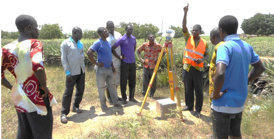
Boundary demarcation with the aim of setting out the project perimeter in the field within one of NEK's wind project areas, Ghana
